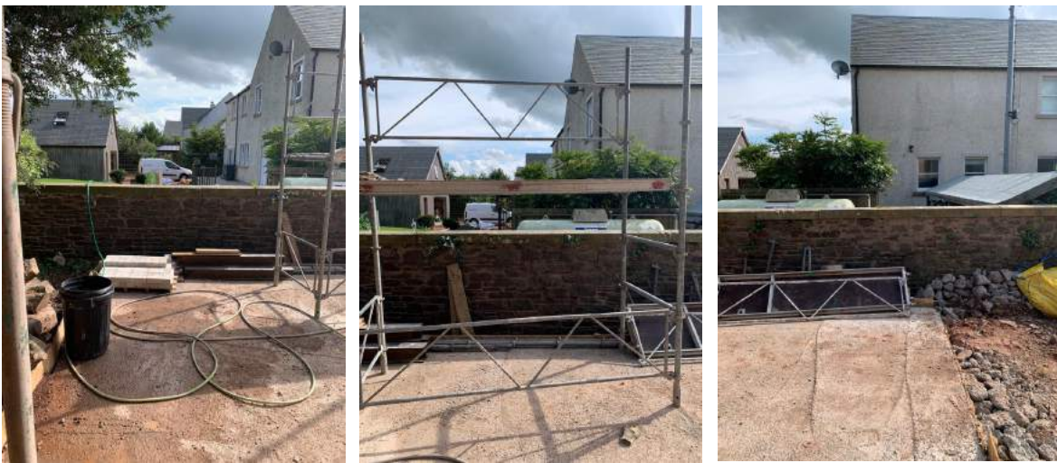
4 Obstructed views from left-, centre- and right-hand sides of the proposed sliding door position.
